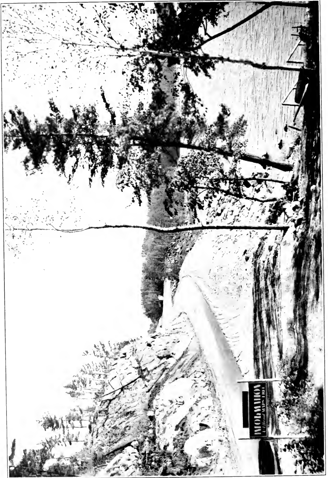
GRADING, HIGHWAY No. 70 - FILL, AT LAKE OF THE WOODS, NORTH OF NESTOR FALLS
